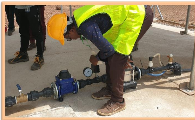
Photo 6: Studying the solar irrigation pump is vital
