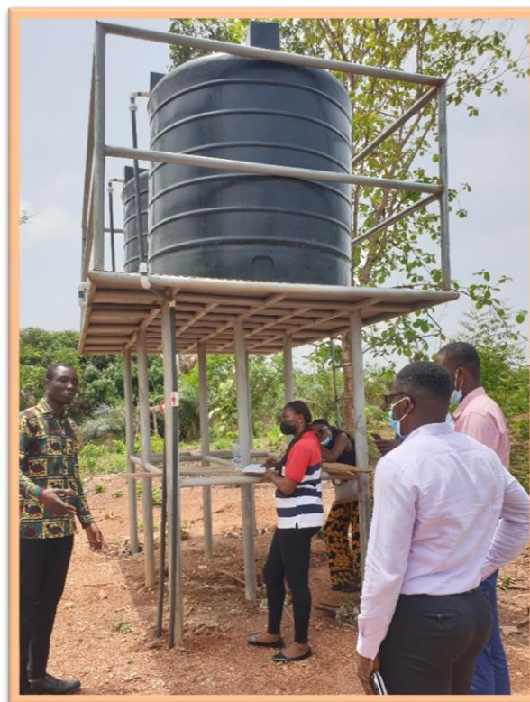
Photo 7: A water reservoir tank on an elevated platform
